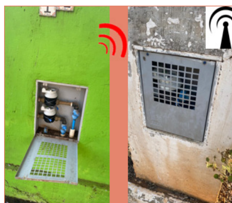
Figure 4: Image of the water meter installation in a double box in the Bueno de Andrada District
